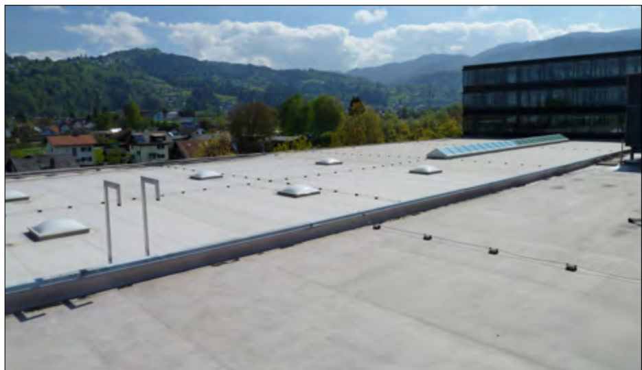
Fig. 3: Overall view of the roof of the Meusburger Building in Wolfurt (Austria)
