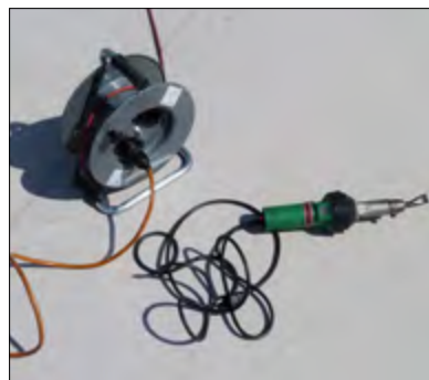
Fig. 6: Hot air welding of new to existing membranes ( Sarnafil® TS 77-18 ) Meusburger Building in Wolfurt (Austria)
